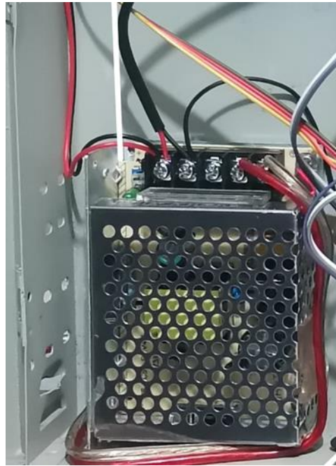
Figure 4. Power Supply Testing Power Supply
